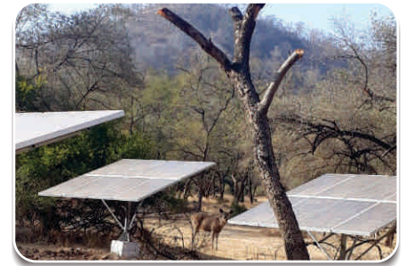
SPV Water Pumping System installed in forest area
